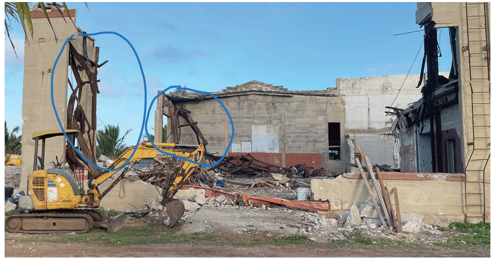
Photos sent to SHPD by Sushil Garg of damaged historic Marconi Wireless Telegraphy Station building after roof collapse.
