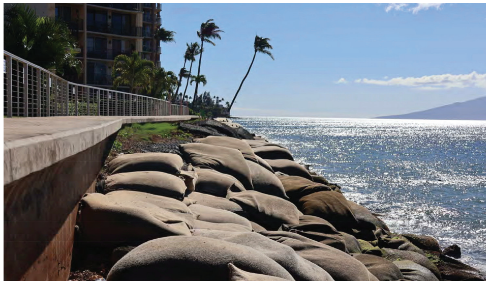
A temporary sandbag revetment fronting the Hololani Resort Condominiums on Maui. CREDIT: DLNR.
