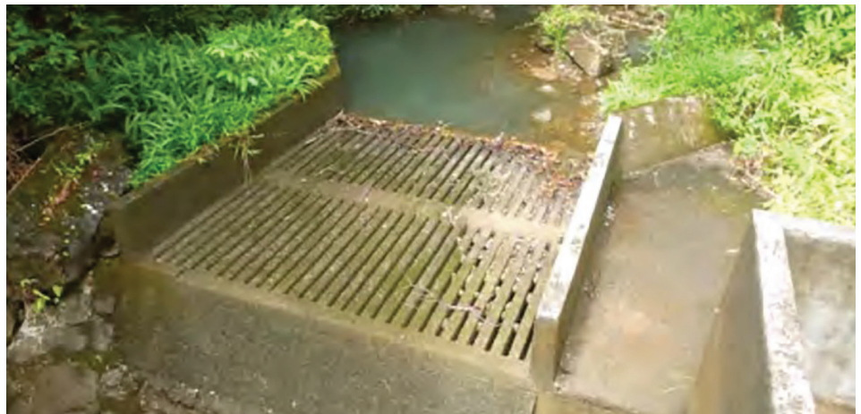
The intake and diversion at Ho'olawali'ili'i stream. CREDIT: CWRM.
