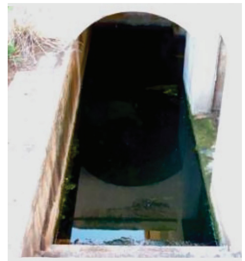
A 2021 survey found that the Marconi hotel’s basement was filled with 4-5 feet of groundwater. CREDIT: HISTORIC STRUCTURES REPORT.
