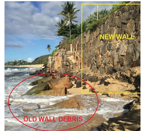
This unauthorized seawall must be removed by the end of this year. CREDIT: DLNR.
